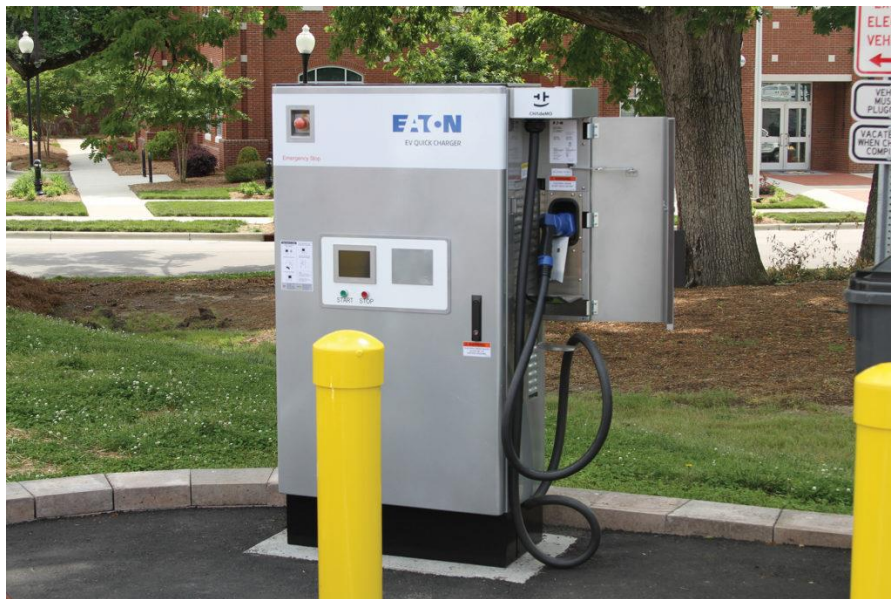
Electric vehicle charging station in Apex, N.C. (Photo courtesy Wake Electric Membership Corporation)
