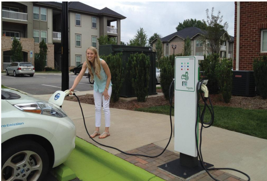
A charging station in Raleigh, N.C. (Photo courtesy Advanced Energy)
